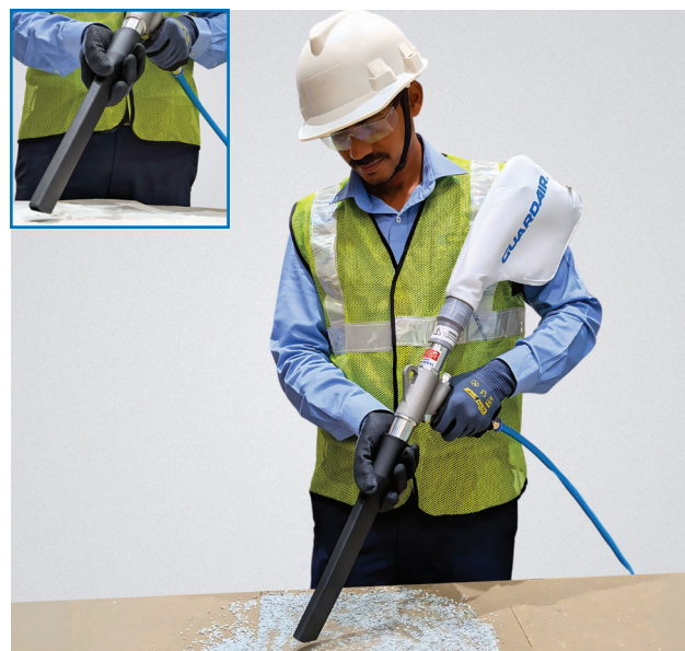
STEP 5 Start Vacuuming - Use the vacuum gun to collect dust, powder, debris or metal chips.
